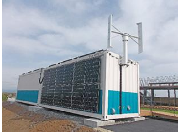
Adopted as an independent power supply for the Flood Prevention Center (Yoshida Town, Shizuoka Prefecture)
