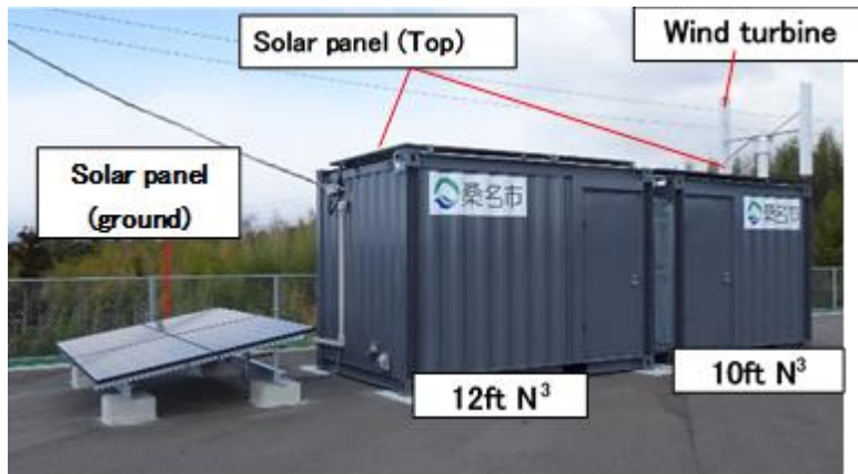
Adopted as an emergency power supply and temperature-controlled storage for disaster prevention base facilities (Kuwana city, Mie Prefecture)
