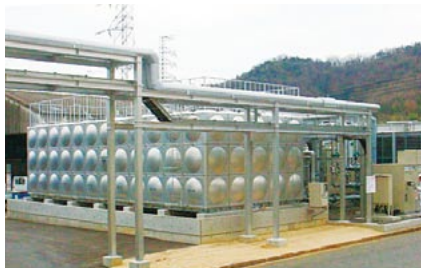
Thermal storage tank for hydrate-slurry air conditioning system (Okayama Works)
