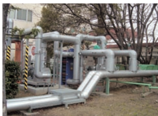
Warm-water discharge pipeline and heat exchanger at Iwata Works (Shizuoka)
