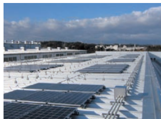
Photovoltaic power generation (Mie)
