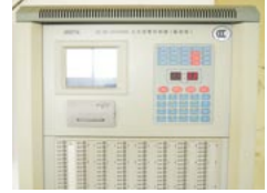
Fire control system
