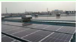
Kuwana Works (Japan) Introduction of 900 solar panels (Approx. 340,000 kWh/year)
