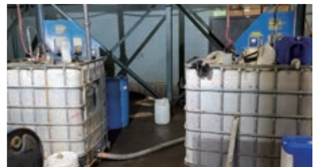
Developed hazardous liquid waste treatment equipment
