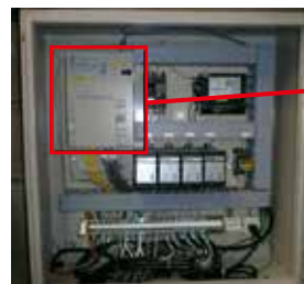
Water monitoring system
