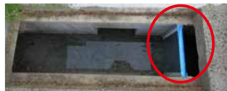
A mechanism was installed at the place between the ditch and the oil separator for disconnecting the outflowing path and collecting oils.
