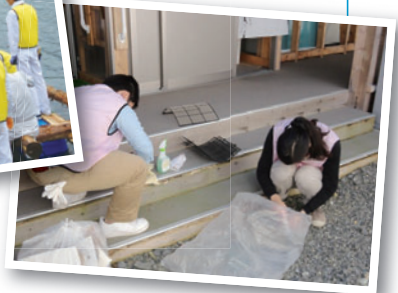
Cleaning air conditioner filters at a temporary housing complex
