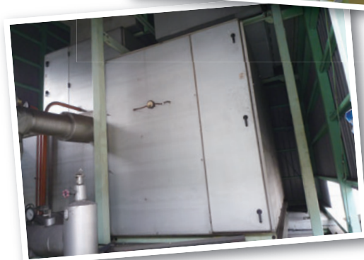
Air handling unit at NTN KINAN CORP.
