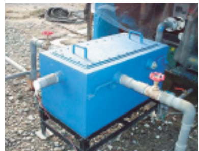
Groundwater purification equipment
