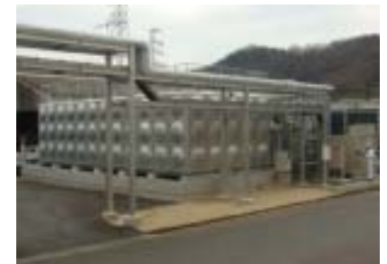
Thermal storage tank for hydrate-slurry air conditioning system (Okayama Works)
