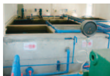
Wastewater treatment unit
