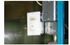
Motion sensor that controls lights
