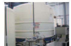
A central coolant control tank
