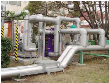
Wastewater pipeline and heat exchanger
