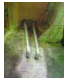
Piping for decontamination
