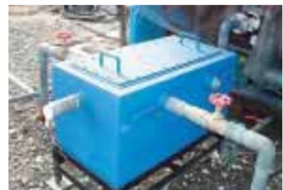
Ground water remediation equipment
