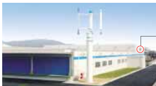
Wind power generator
