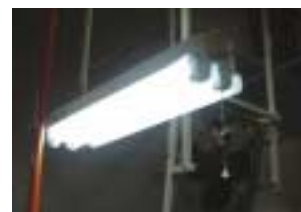
Fluorescent light with pull switch
