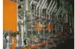
Heat treatment furnace converted to run on natural gas
