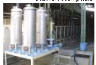
Reusing rainwater as heat treatment cooling water
