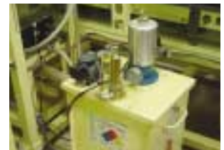
New rust inhibiting oil supply unit
