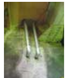
Piping for decontamination
