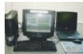
Demand Control System that conducts centralized control of air conditioning packages
