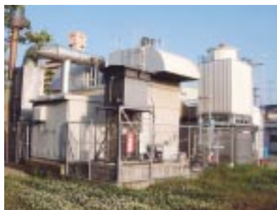
Co-generation facilities (NTN Powder Metal Corporation)
