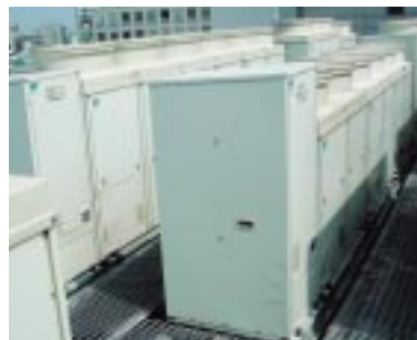
Ice storage air conditioning system
