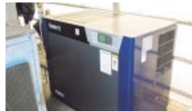
Compressor with inverter 75kW
