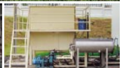
Wastewater treatment equipment
