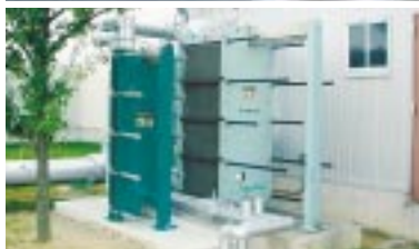
Heat exchanger to use co-generation exhaust heat
