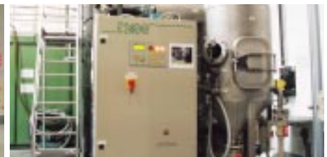
Oily water separator
