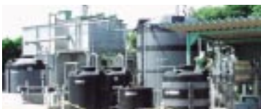
Sewage treatment facilities
