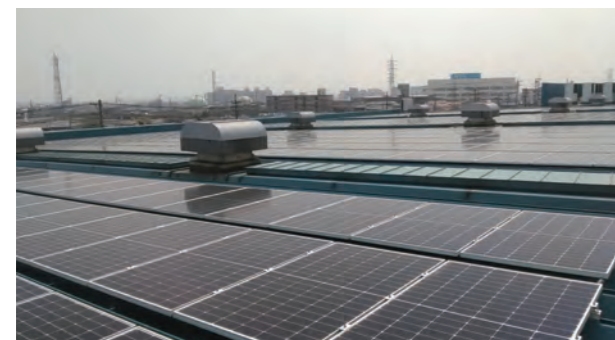
Kuwana Works east wing of its extra-large bearing plant
