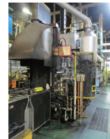
Okayama Works City gas burner heating type furnace
