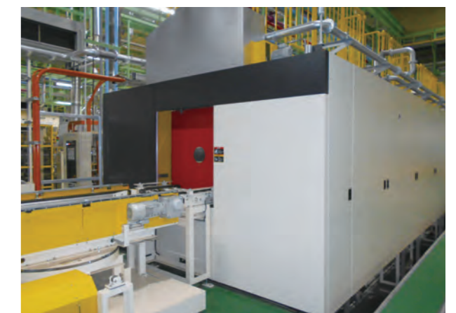
Kuwana Works Electrically heated vacuum carburizing furnace
