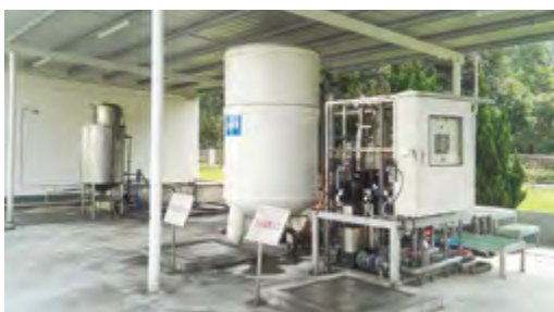
New sewage treatment facility
