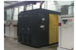
High-efficiency compressor at NTN BEARING Mfg CANADA
