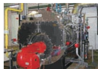
A boiler at SNR that was converted to run on natural gas
