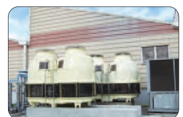
The water-cooled chillers for the compressor at Okayama Works
