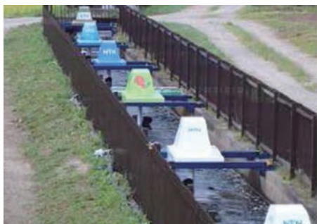
▲ NTN micro hydro turbines placed in series in the same conduit
