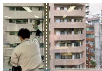
Energy-efficient dual-pane windows installed in the head office At left: with dual panes installed At right: Before dual-pane installation with low-E coating
