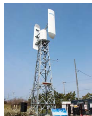
NTN Vertical Axis Wind Turbine (10 kW)
