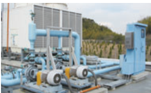
Cooling water pump converted to inverter type
