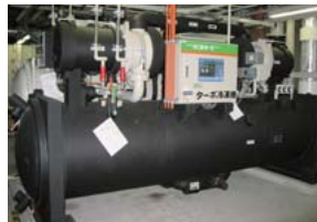
High-efficiency turbo chiller (Nagano Works)
