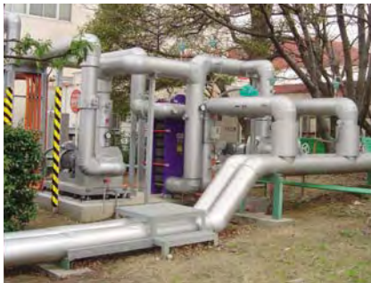
Wastewater pipeline and heat exchanger
